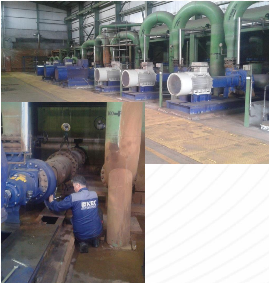
SABA pump station
